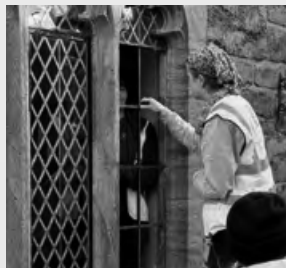
Window repair at The Almshouse of St John the Baptist & St John the Evangelist, Sherborne
